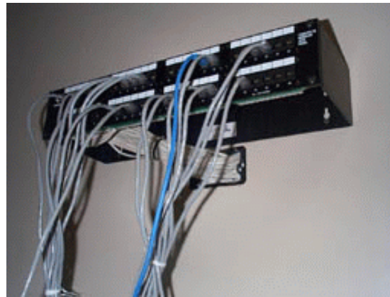
48 Port Patch Panel
