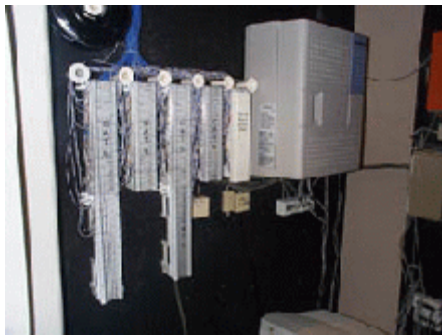
Telephone System Patch Panel and T1 Fiber Connection Box
