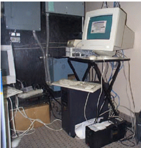
Network Server Closet
